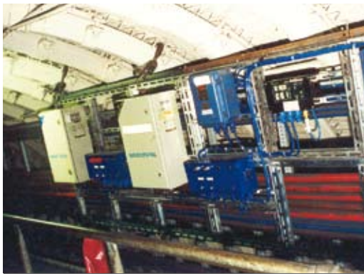
Equipment for measuring ventilation control underground
