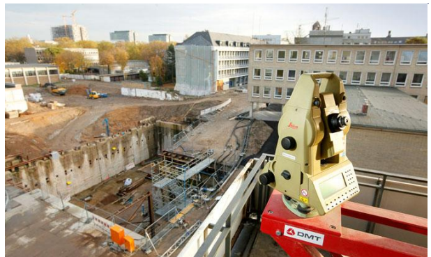
Total station for stability monitoring
