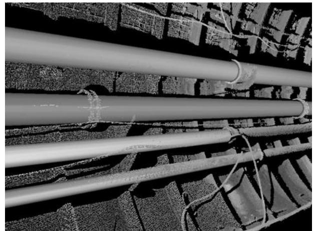
Pipes and tubings
