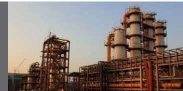
Scrubber and Distillation Columns
