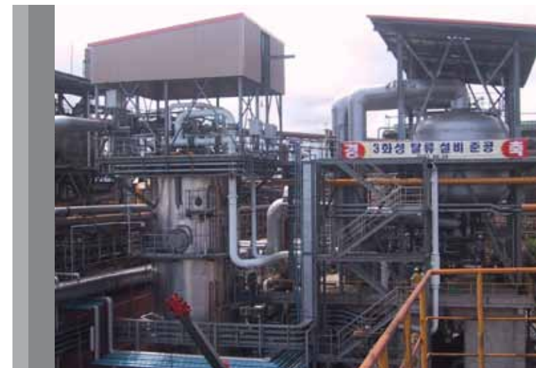
Claus Plant for Sulphur Production
