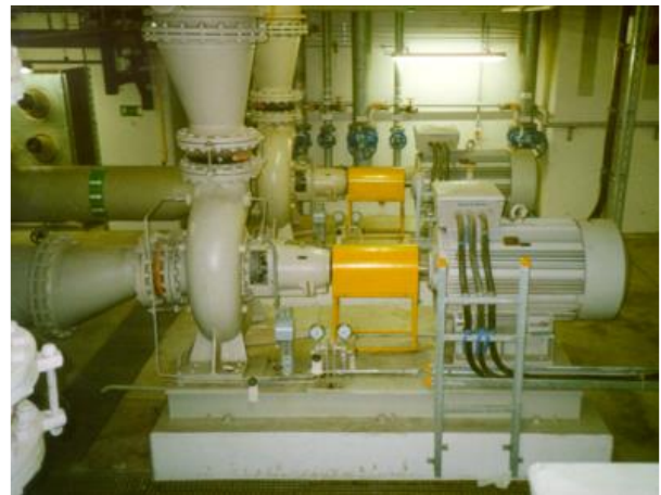
Intermediate coolant pumps in the water circuit of 800 MW brown coal power plant
